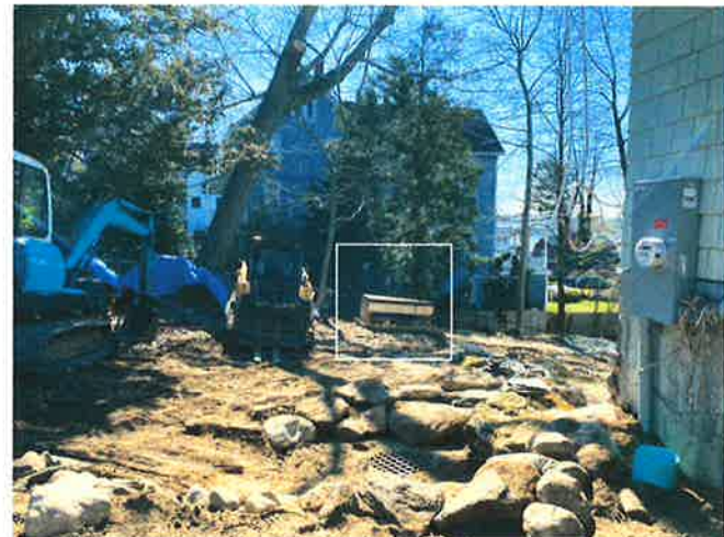
LOOKING WEST ACROSS FRONT YARD TOWARD BATHWAY STEPS & SOUNDVIEW APARTMENTS SHOWING GENERATOR PLACEMENT
